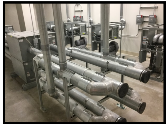
Level B Pneumatic Tube Room
