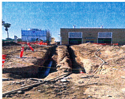
Domestic and Fire Water Lines
