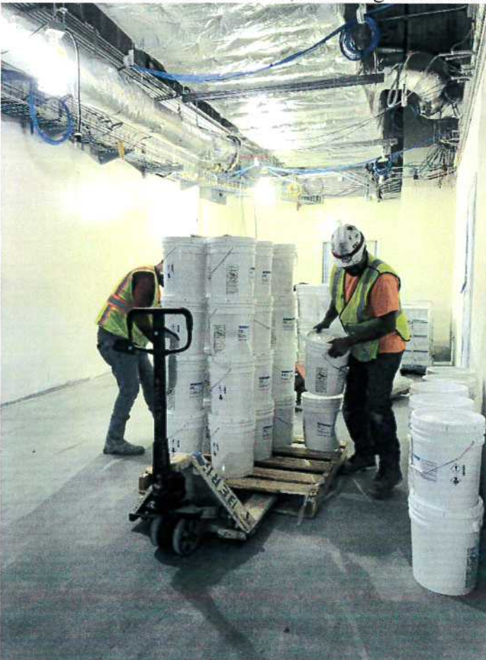
Sterile Core South: Finish floor prep complete; workers unloading finish flooring materials. Prepared by: Kate Herring
