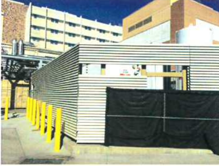
Bulk O2 Yard Enclosure
