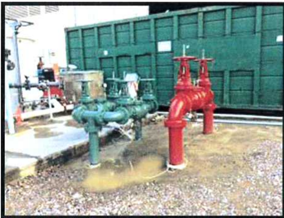
Helix Water Lateral Line
