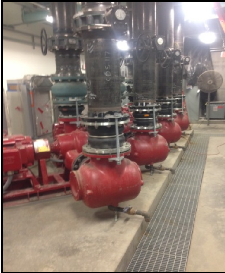
Flex Connectors on 500 HP Pumps
