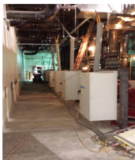
VFD's for the Pumps
