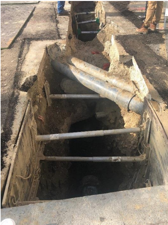
9-28-18 Helix Waterline Trench: PVC lines are control/monitoring for diesel generators. Behind them is an encasement for electrical lines.
