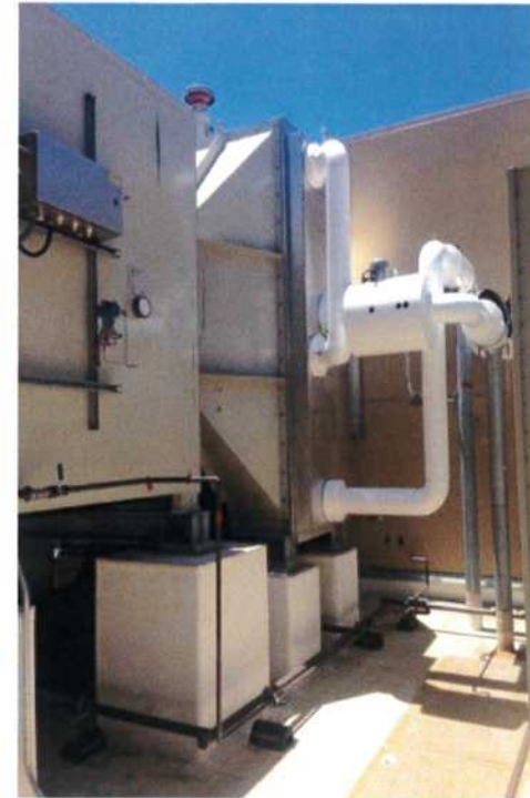
Low Roof Turbine Inlet Cooler
