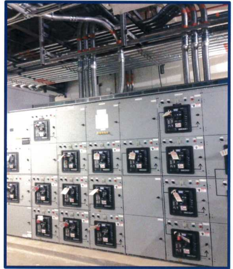
Switch gear is now energized
