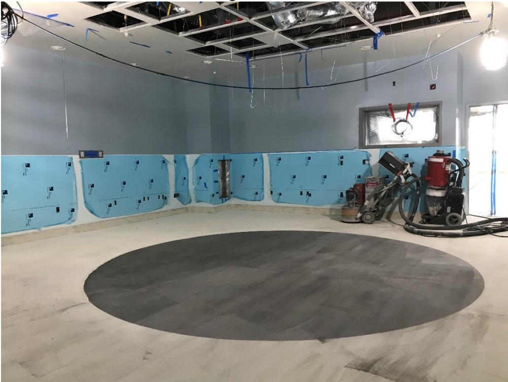
11-13-17: OR #1027 (Open Heart OR) Drywall ceiling installation complete; wall protection complete; sanding before final coat of resinous flooring.
