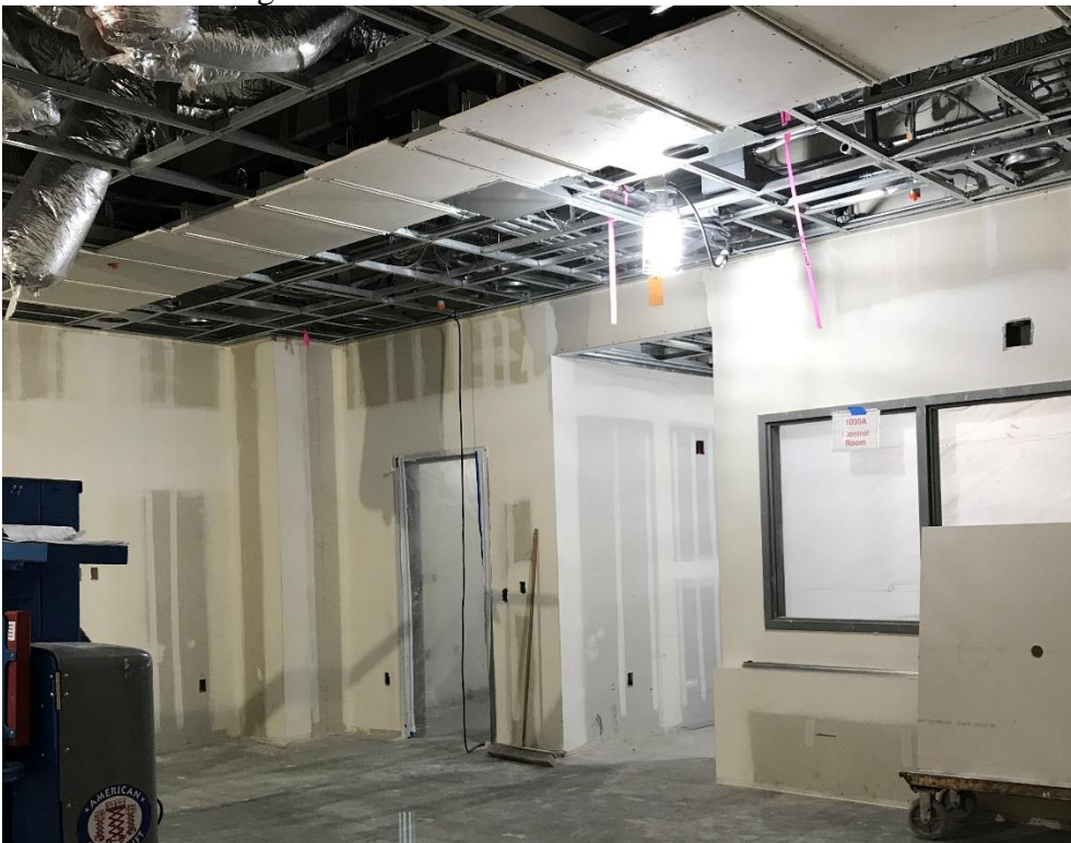
10-24-17: OR #1030 (Hybrid OR) Drywall ceiling installation in progress. Prepared by: Kate Herring
