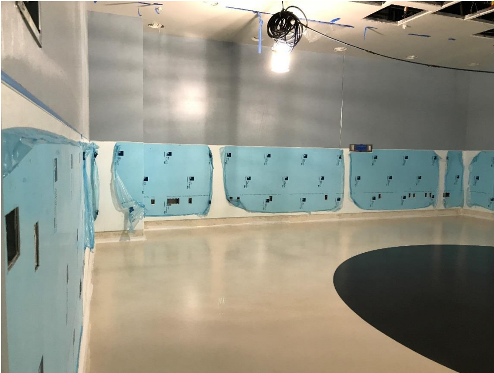
11-16-17: OR #1025 (General OR) Painted. Wall protection, flooring complete, ready for installation of finish electrical and mechanical grilles.
