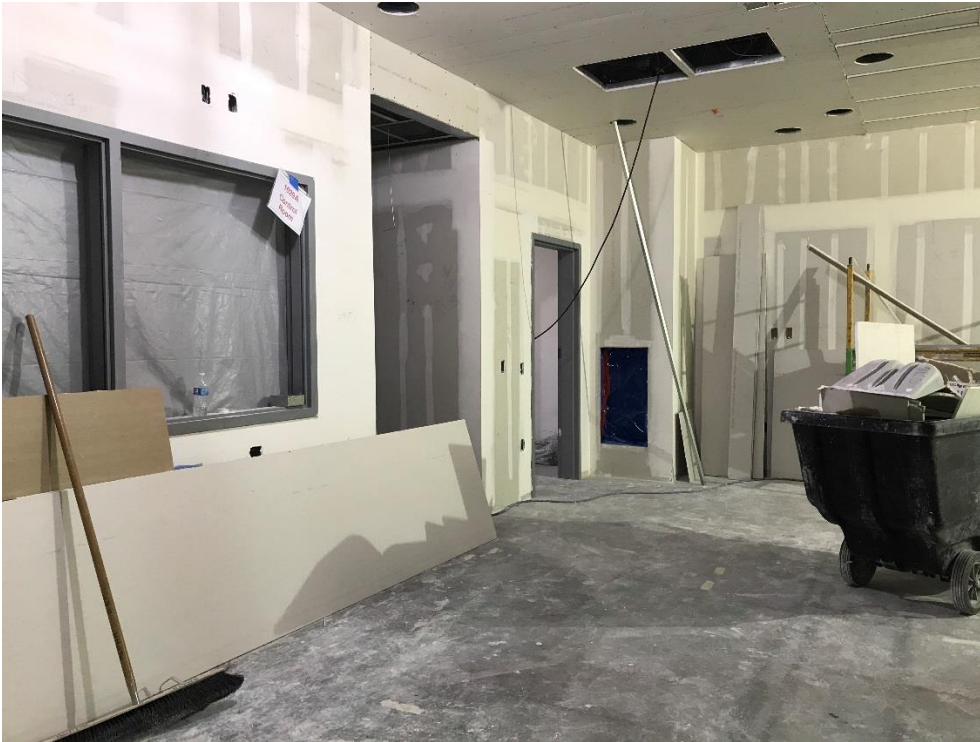
11-16-17: OR #1029 (Hybrid OR) Ceiling drywall complete; ready to paint and install wall protection, with finish flooring to start 12-4.
