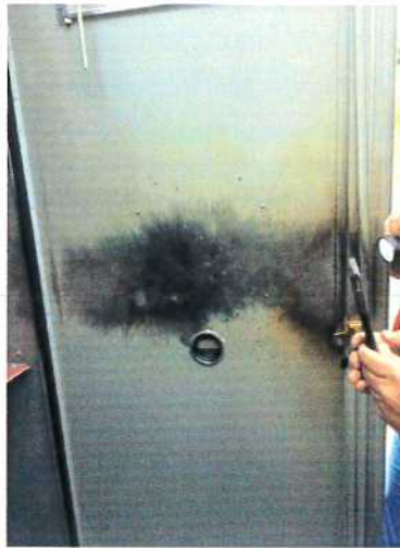
Evidence of Electrical Short on "Rule 21" Door
