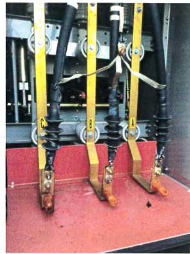
Damaged bus fingers inside Rule 21 Gear
