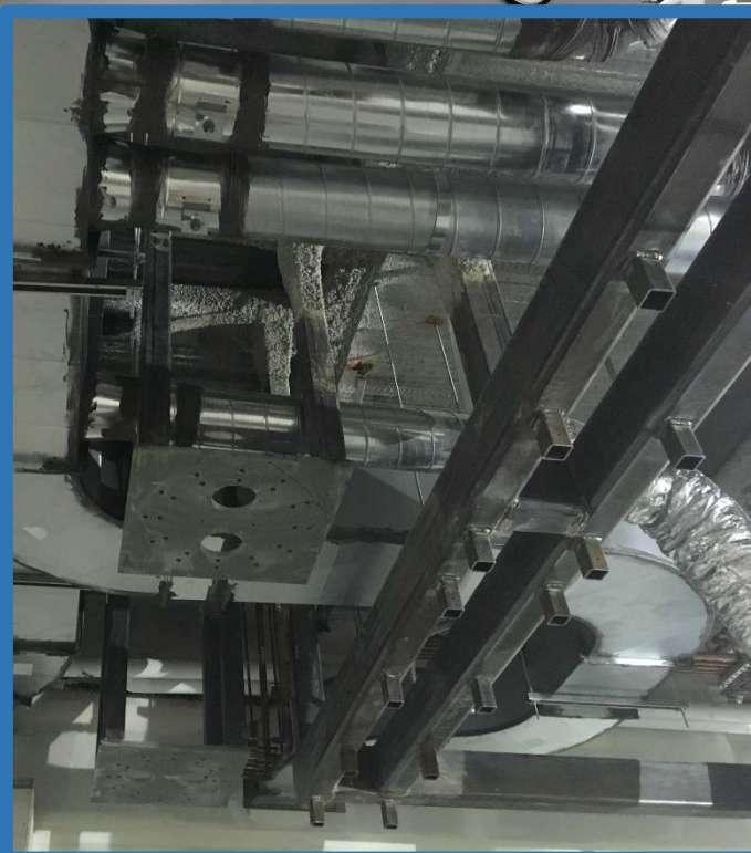
Looking back: Ductwork, Overhead structural supports in Hybrid OR #1030
