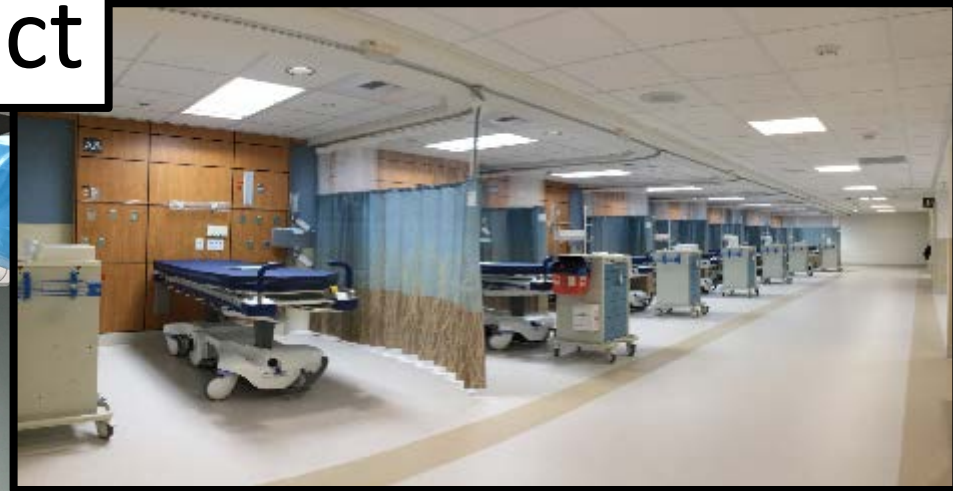
Gurney, curtains installed in new PACU
