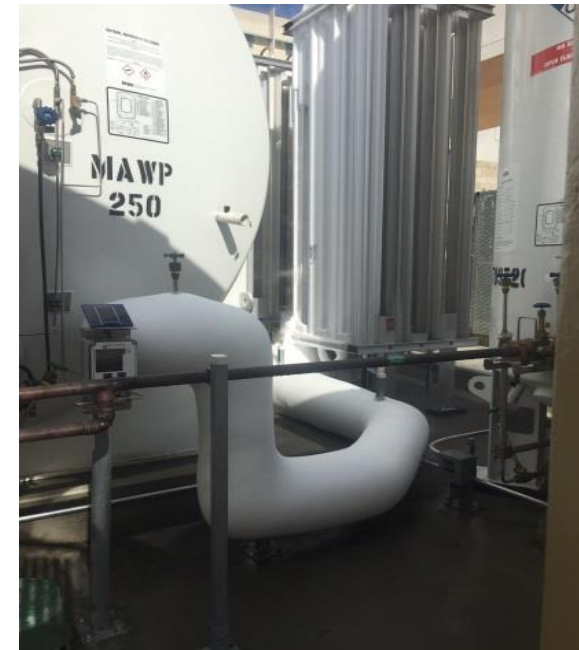
Bulk O2 Equipment In Operation
