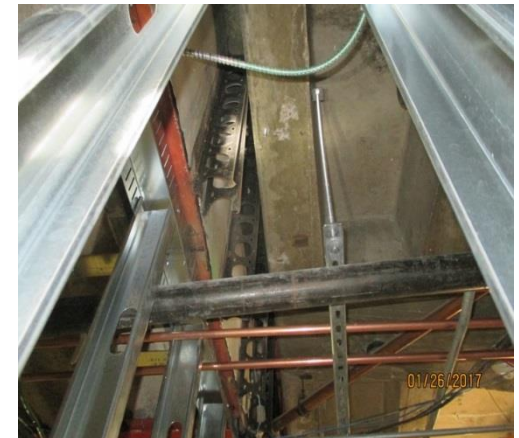
Gaps in fire separation walls
