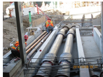
Piping in Utility Tunnel
