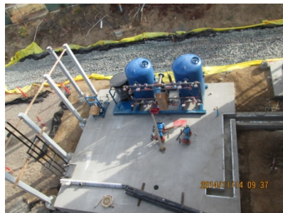
Chemical Yard Pad and equipment
