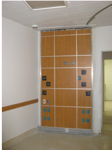
Photo #4: Patient Headwalls
