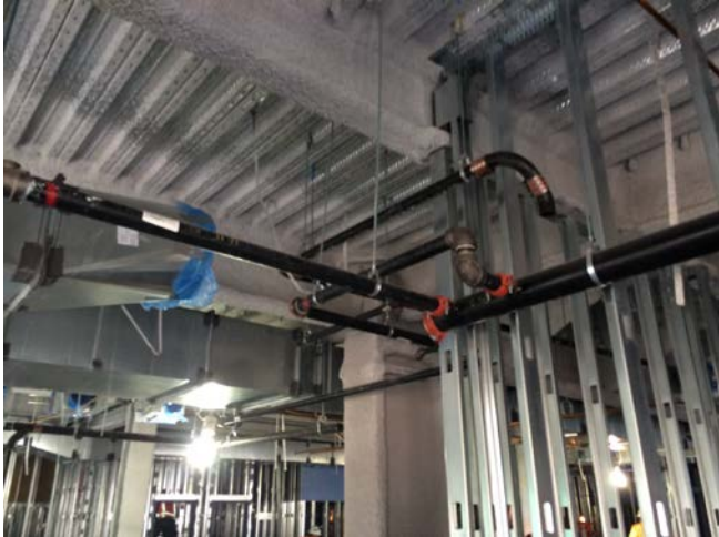
• Level A Overhead Fire Protection
