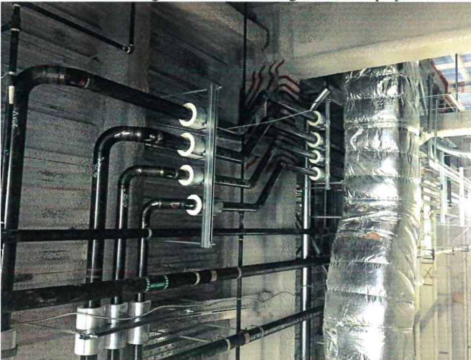
Domestic hot and cold water piping connecting to the Infill project.
