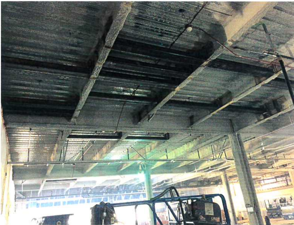
Structural Steel installation in the operating rooms at the South end of the project, above ORs #1027 & #1029
