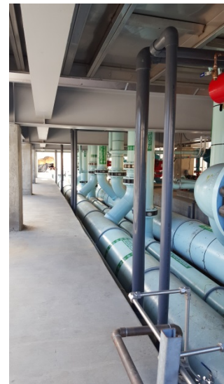
Cooling Tower Pipe System
