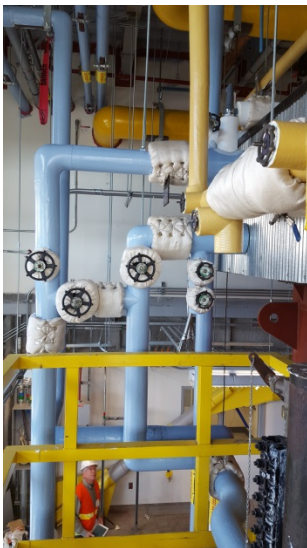
Chill Water Pipe System
