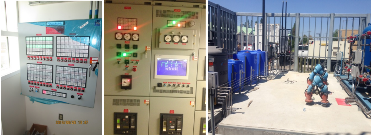
Remote Annunciator Panel in Control Room
