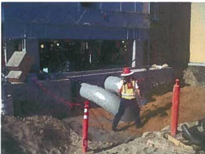
Cooling Tower Chilled Water Piping
