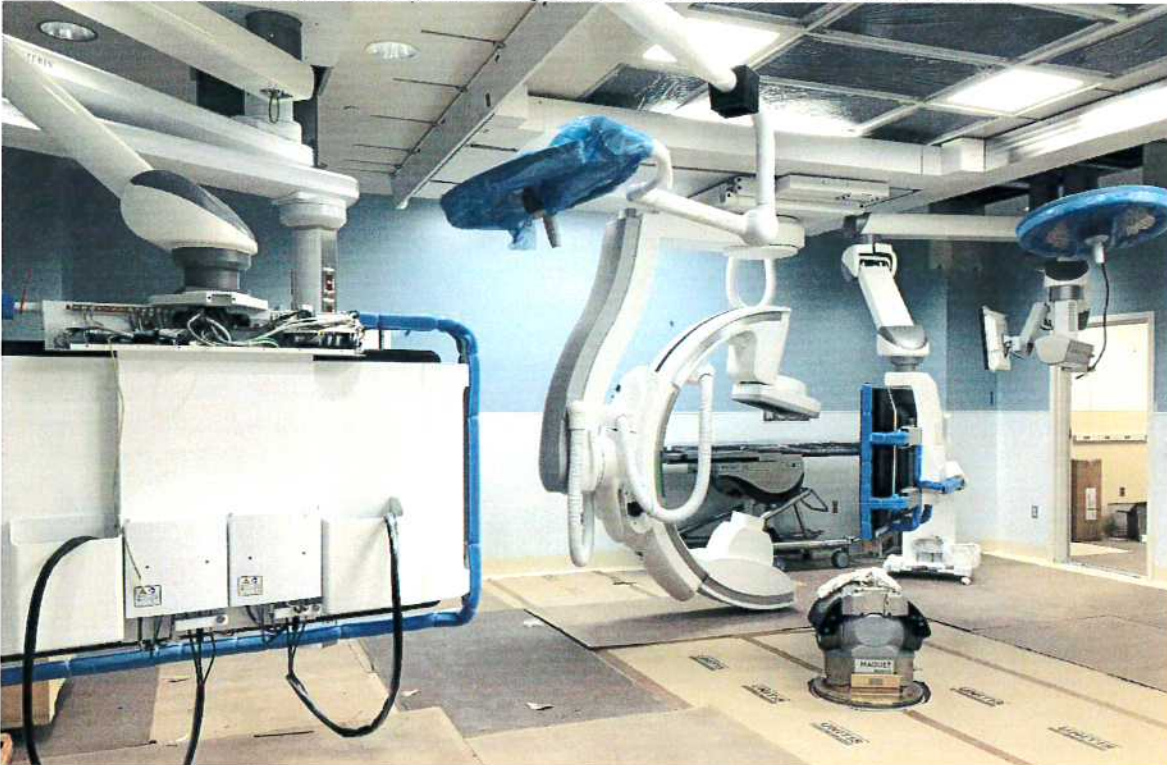
3-15-18: OR #1030 (Hybrid OR) Medical equipment installation nearing completion, including all booms (lights, monitors, anesthesia), C-Arm and Maquet Table base.
