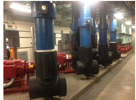
Chilled Water pumps
