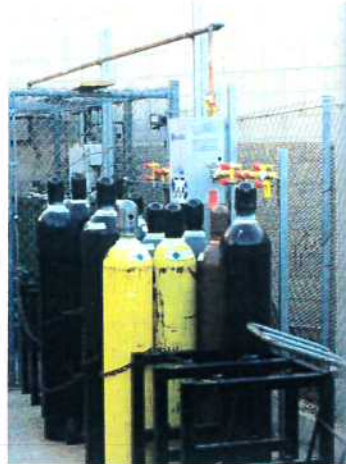
Nitrogen and nitrous oxide manifolds
