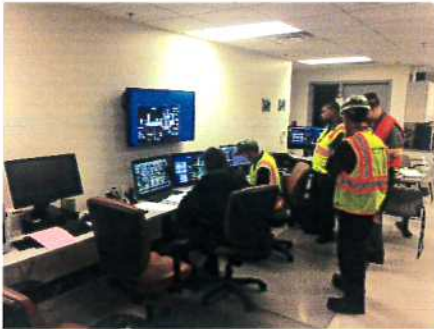
L5 Test – From the new Control Room
