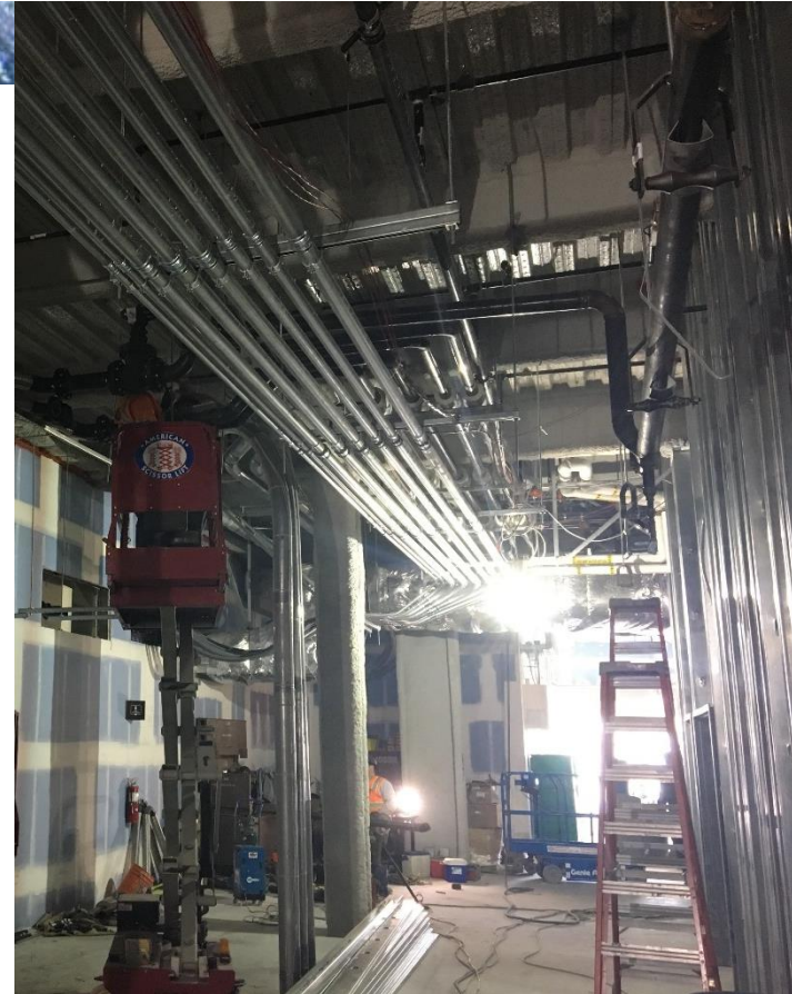
West corridor of the Build Out: Conduits for the tie-in to the Infill Project
