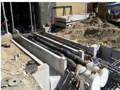
CEP to CEP Vaults Chiller and steam lines
