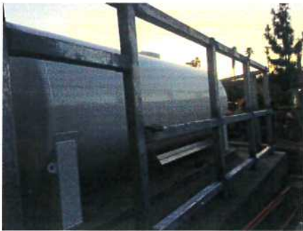
New O2 tanks, vaporizers, and SS for louver wall
