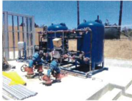
Soft Water skid
