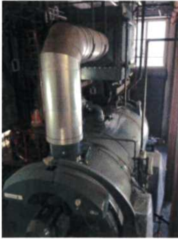
Boiler and associated piping
