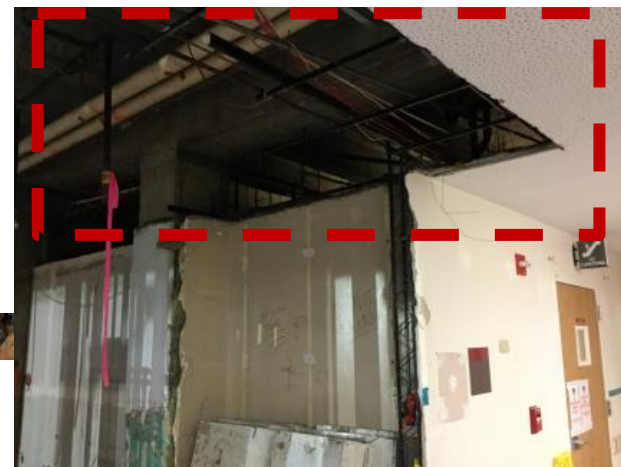
Existing Stairwell is not properly rated to ceiling:
