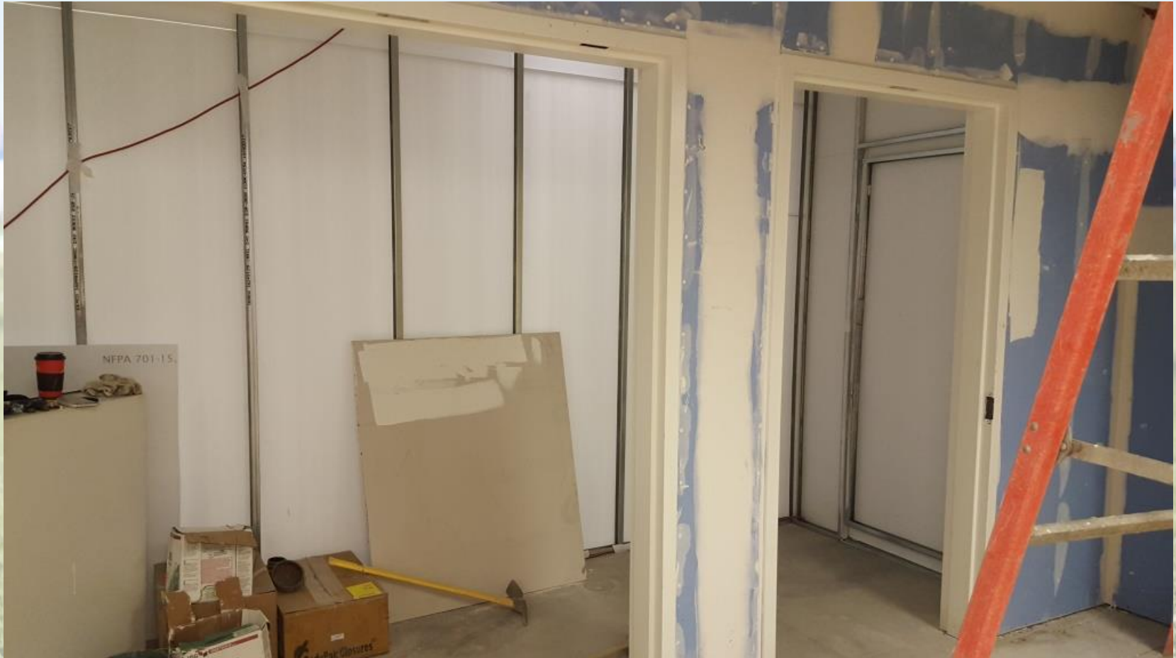
Level B "Punch Through" in EVS Closet
