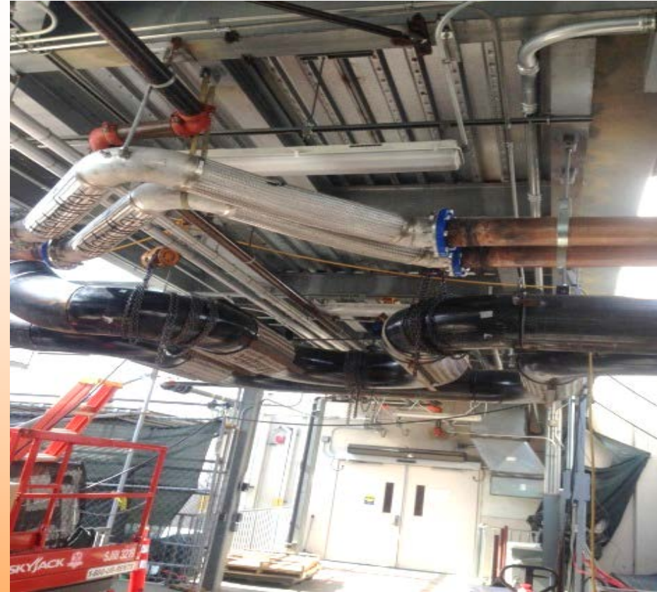
Piping going to Trellis
