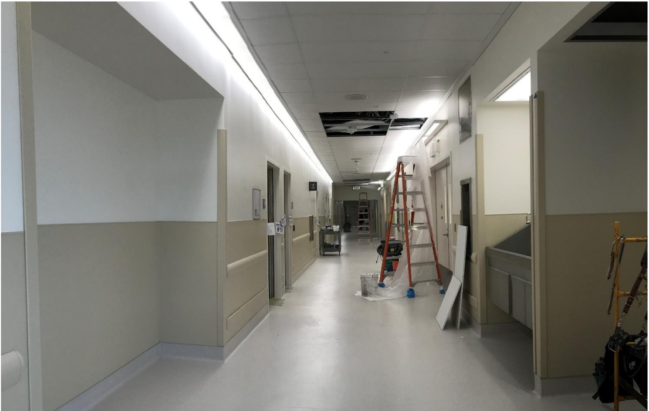
6-13-18: West Corridor: Chasing leaks in the humidification system.
