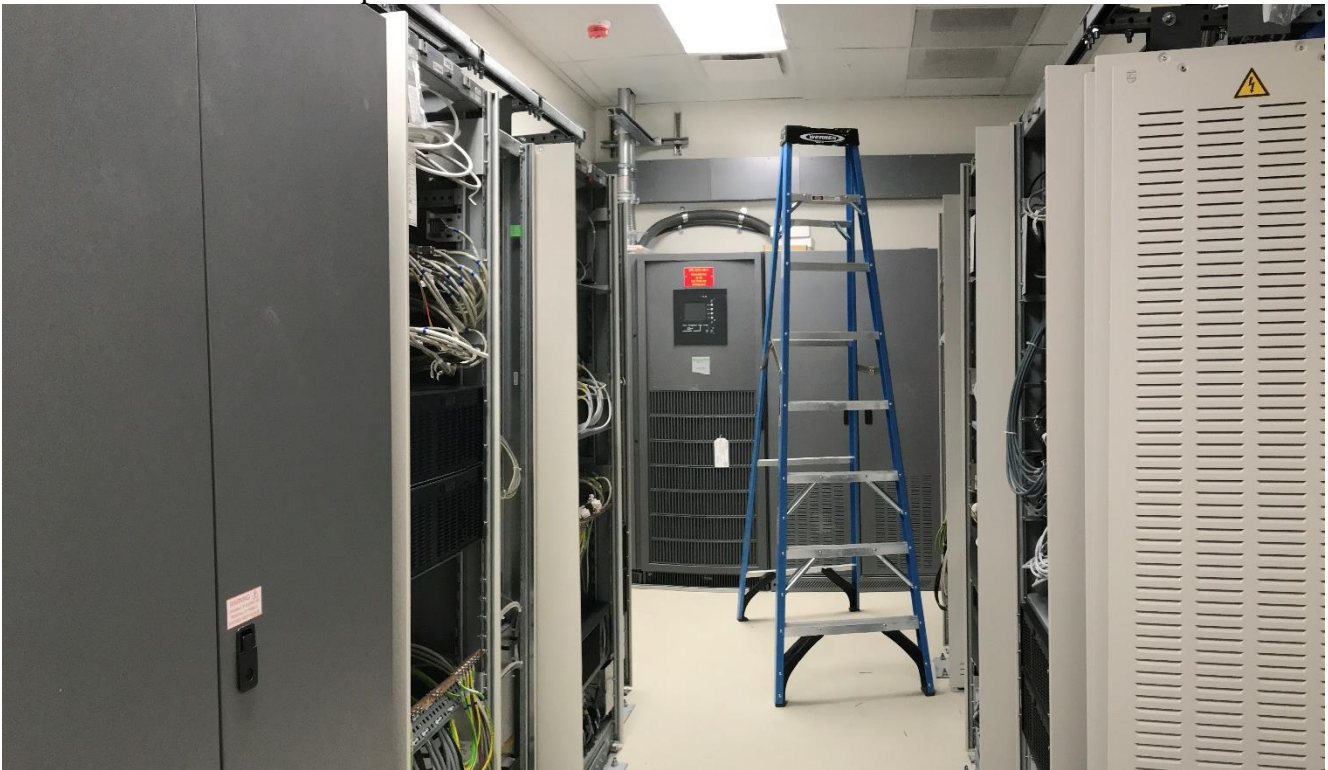
6-13-18: Typical Equipment Room (1023B) cabinets open and work by medical equipment providers in progress.
