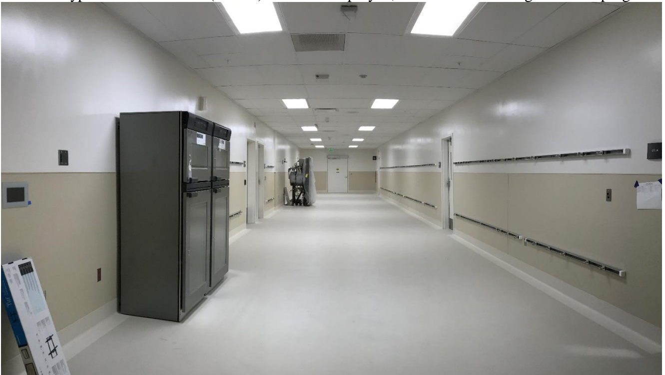
6-13-18: South Sterile Core: Sterilizer to be installed, warming cabinets anchored but otherwise complete.
