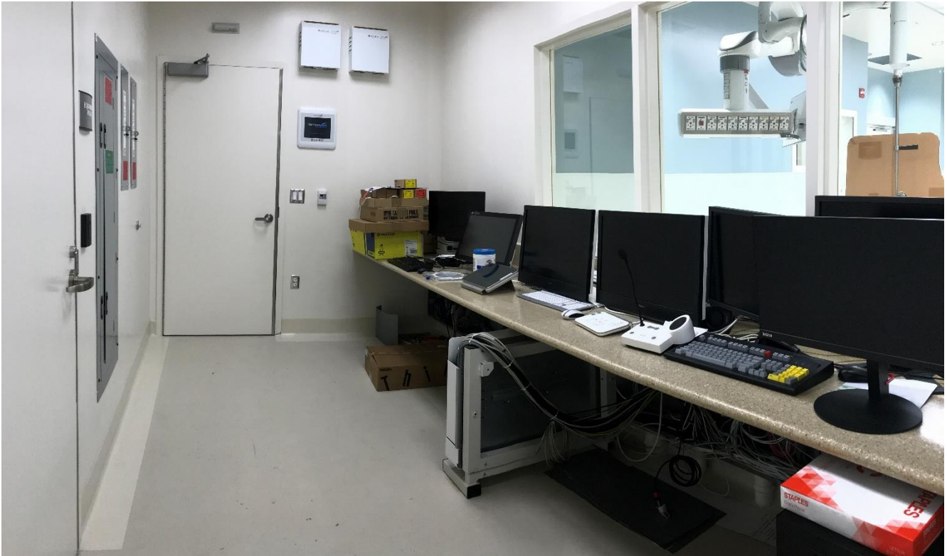
6-13-18: Typical Control Room (1030A): monitors deployed, under-cabinet wiring a work in progress.
