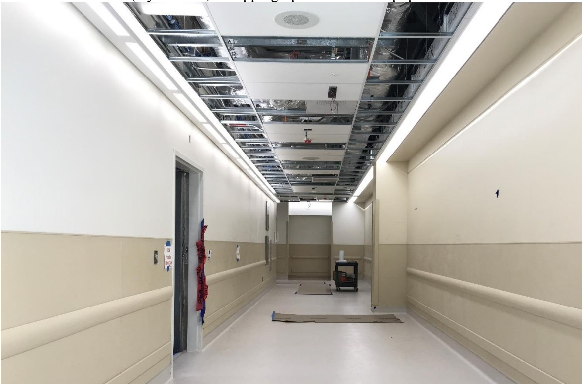
4-24-18: South Corridor: Wall protection, T-Bar grid, flooring, fire sprinklers, smoke detectors installed.
