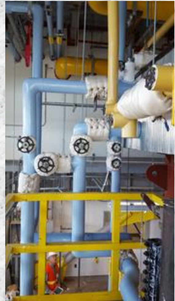
Chill water and steam piping
