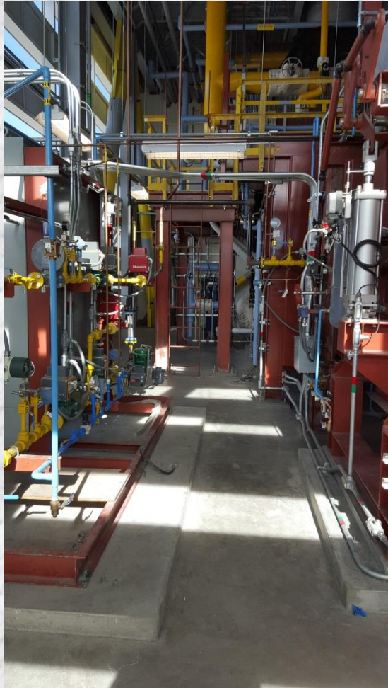
Heat Steam Recovery Generator (HSRG) room
