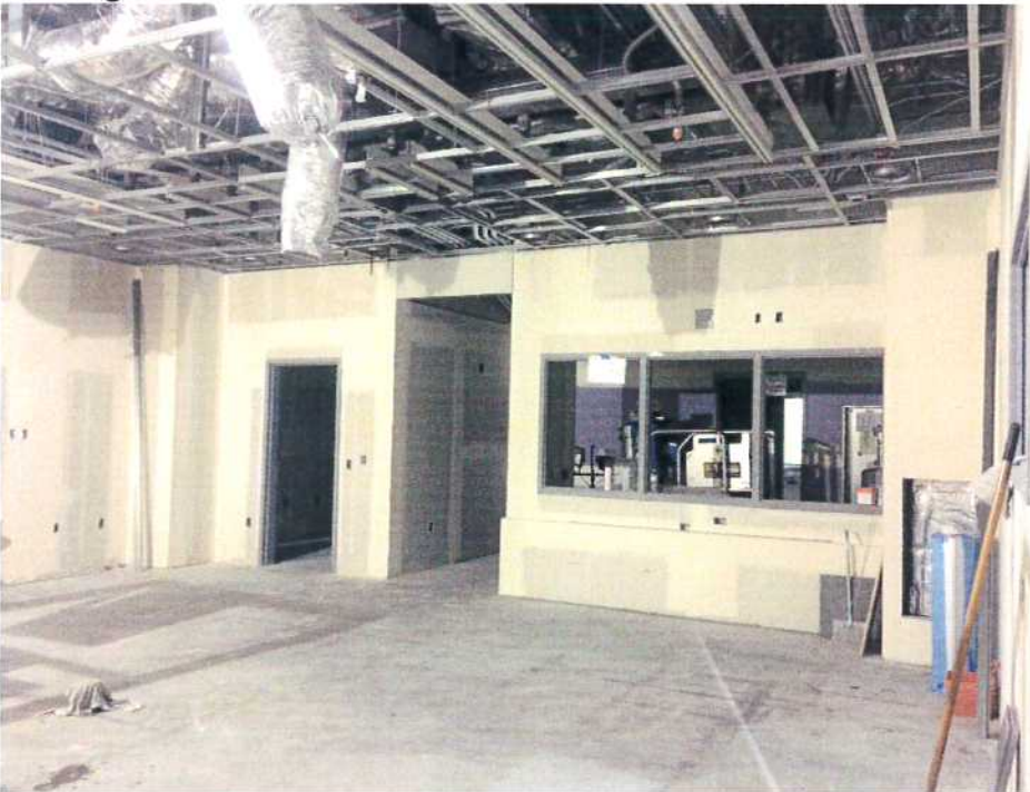
10-24-17: OR #1030 (Hybrid OR) Ready for drywall ceiling installation, pending final above-ceiling cleaning.
