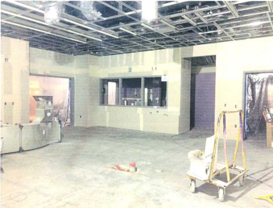
10-24-17: OR #1029 (Hybrid OR) Ready for drywall ceiling installation, pending final above-ceiling cleaning.
