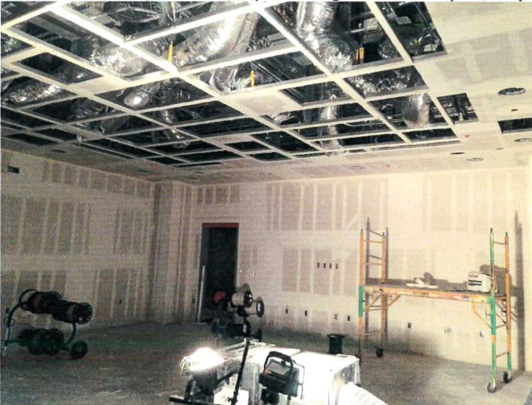
10-24-17: OR #1027 (Open Heart OR) Drywall ceiling installation complete, paint ready pending final mud/sanding.
