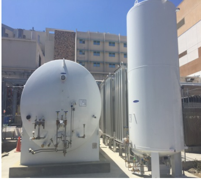
New O2 tanks and vaporizers
