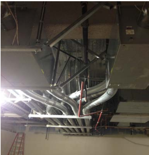
Tube runs to the Blower Room
