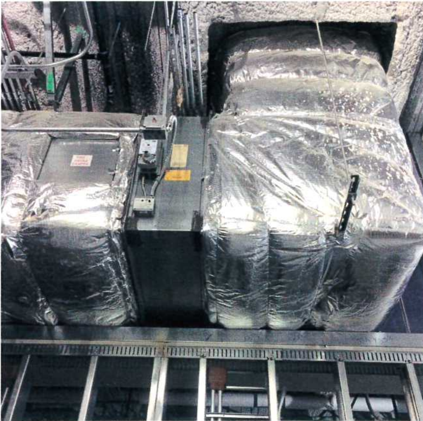
8-16-17: Existing, incorrectly-located 2-hour smoke/fire damper
