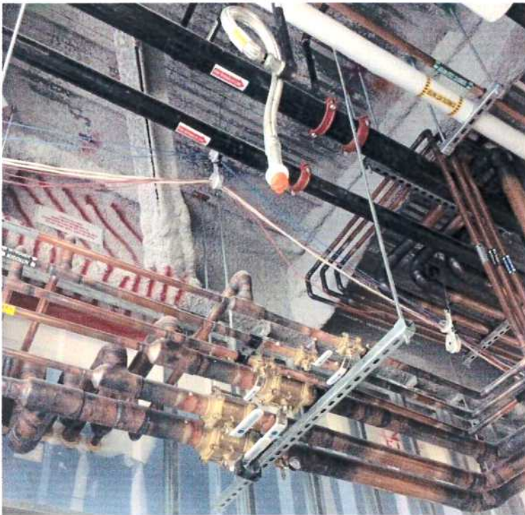
8-8-2017: Relocated (to enable future access) medical gas valves above ceiling, west corridor.
