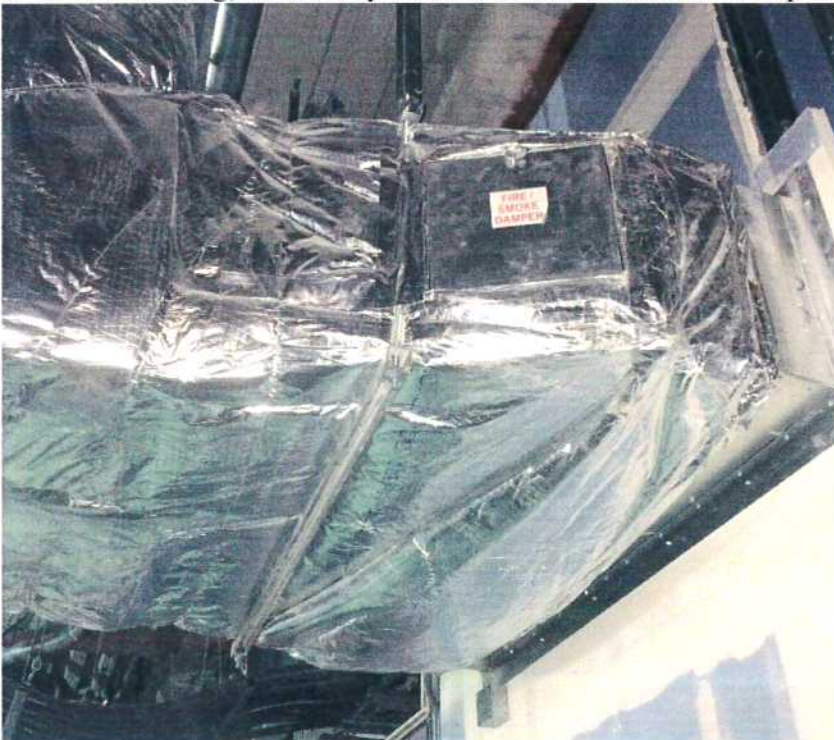
8-16-17: Existing, Insufficiently sized seismic ductwork connection between Build Out/Infill.
