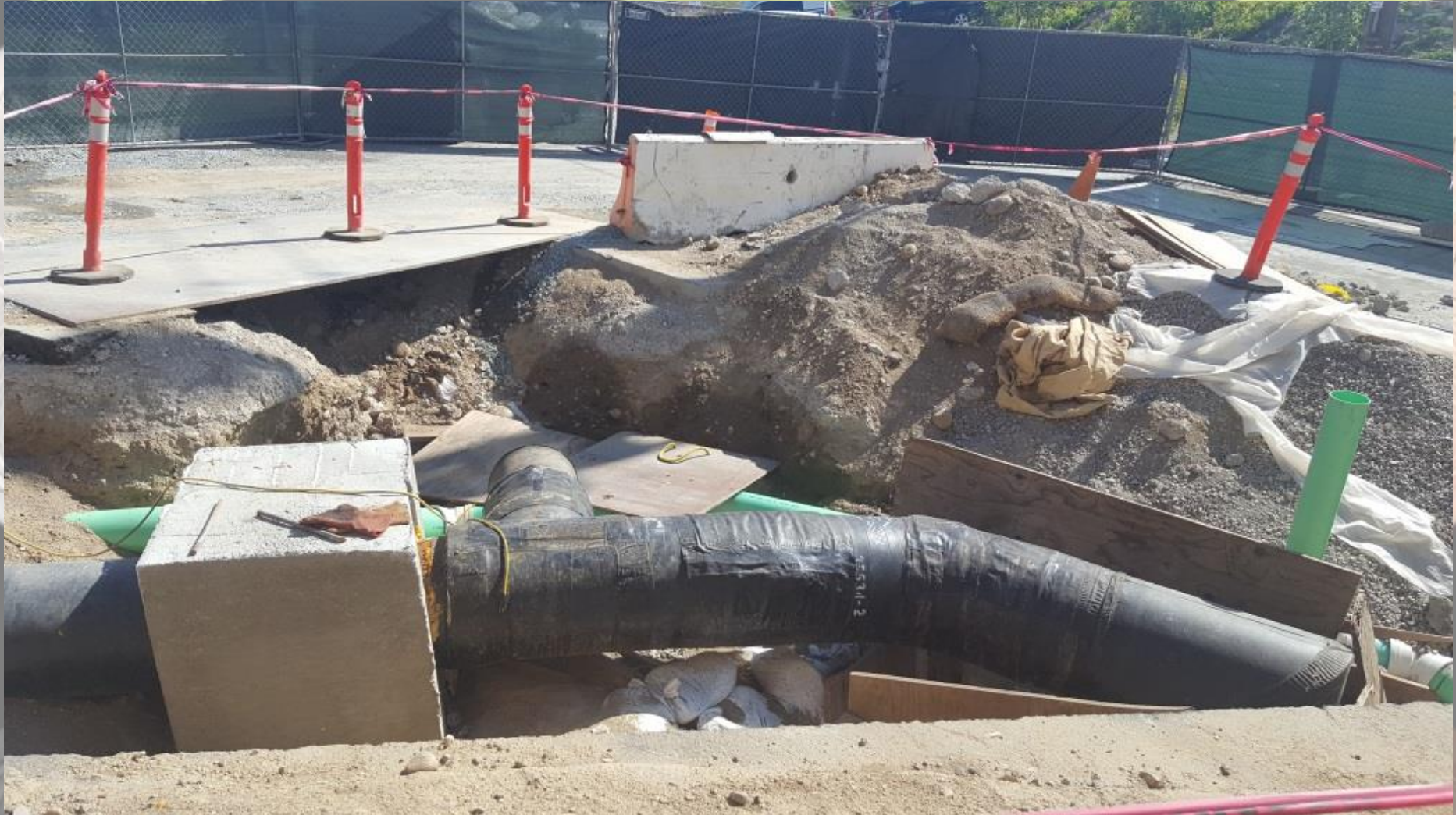
North Steam Line
