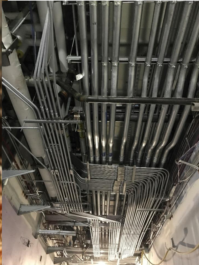
West Corridor #1003: overhead utilities fill the 7 feet of space above the ceiling
