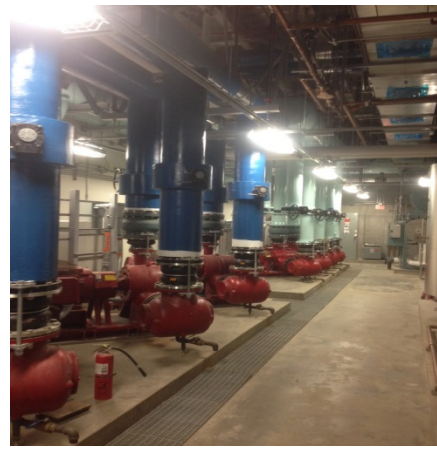
Chilled and condenser water pumps with flex connectors
