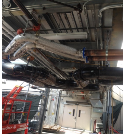
Piping going to Trellis
