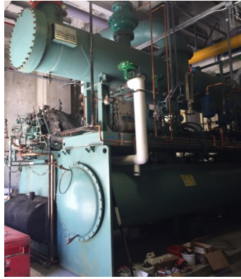
950 Ton Steam Chiller Installed
