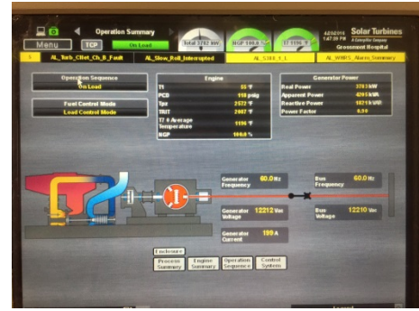
Solar Turbine carrying the campus load at 3.8 MW
