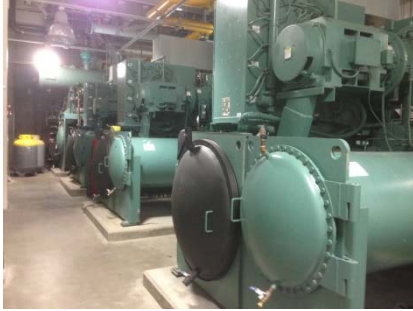
Chiller room with all 4 Chillers installed
