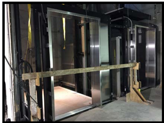
North Elevator Cabs
