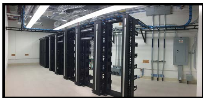
Level B IS Comm Room
