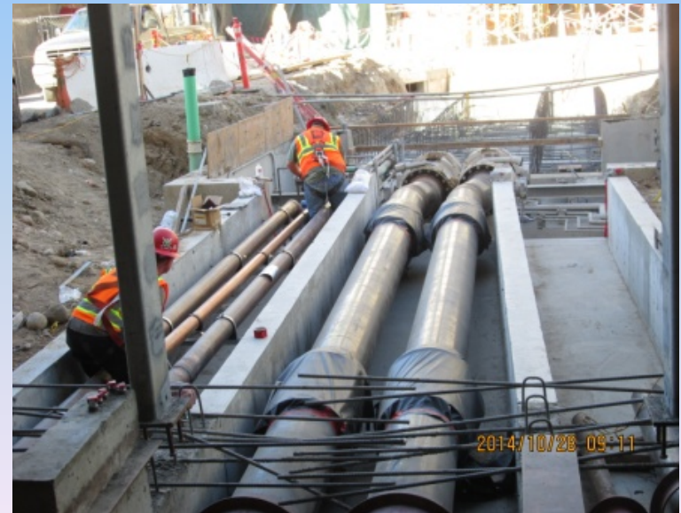
Piping in Utility Tunnel
