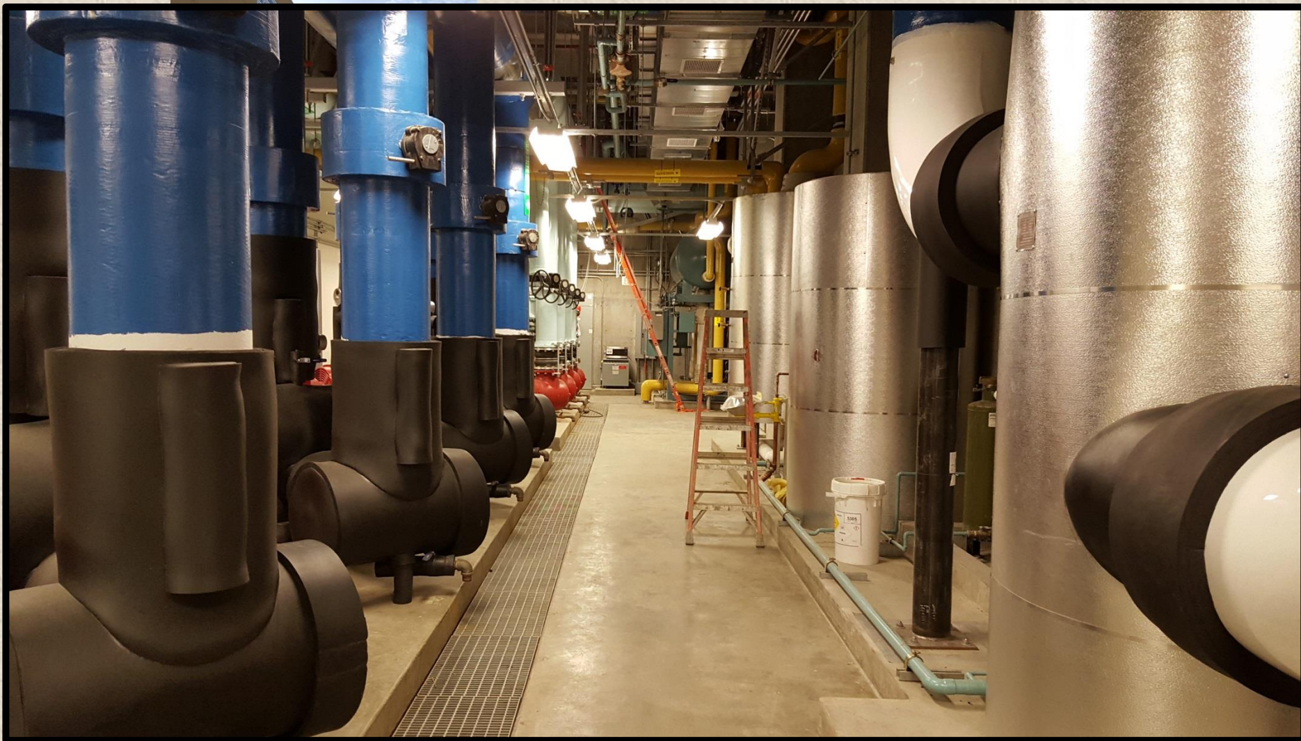
Chilled Water Pumps
