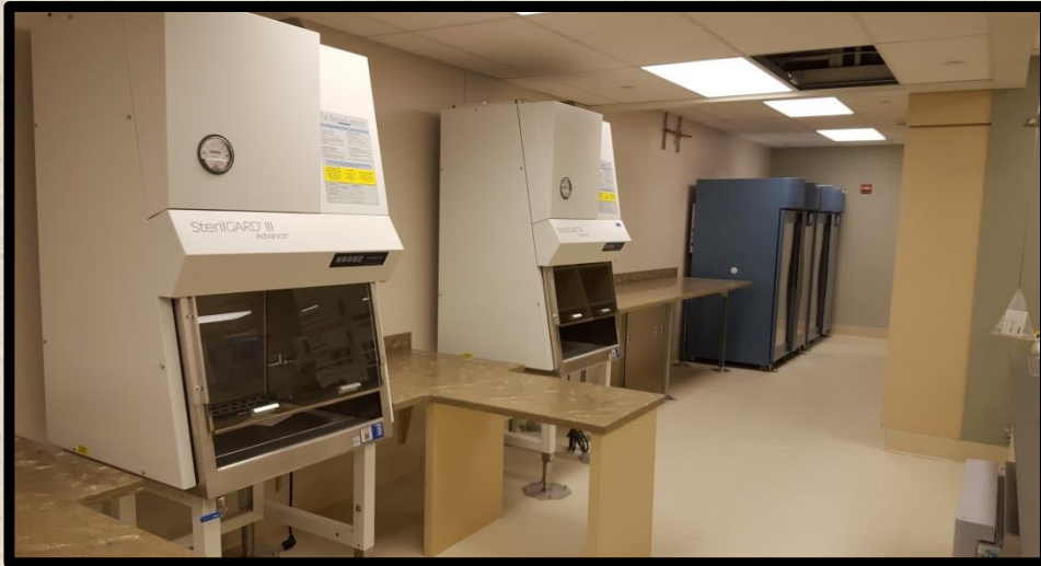
Lab Fume Hoods
