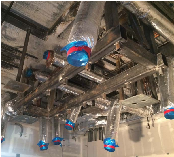
Cath Lab #1023: Mechanical ductwork installation, structural framing to support booms and CT Scanner, med gas lines complete
