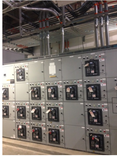
Main Switch Gear Ready For Power
