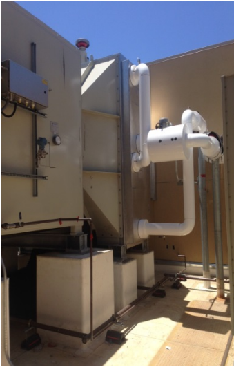
Low Roof Solar Inlet Cooler
