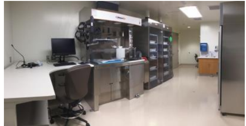
IS equipment installation in Grossing Lab
