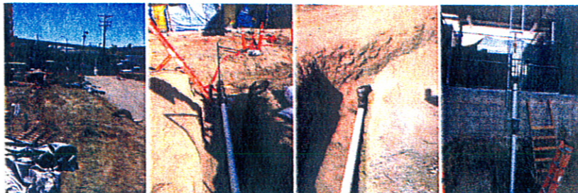
Views of the new steel gas line about to be dropped into the trench.
