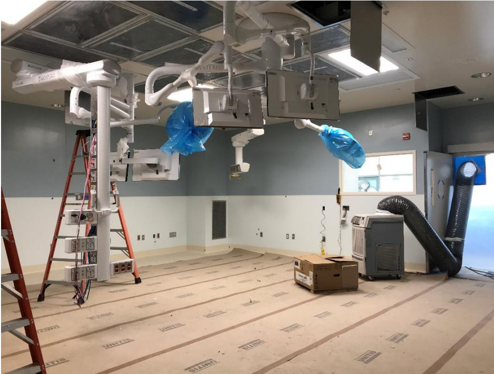
2-20-18: OR #1025 (General OR) Overhead Medical Equipment installed, complete except for final wiring.
