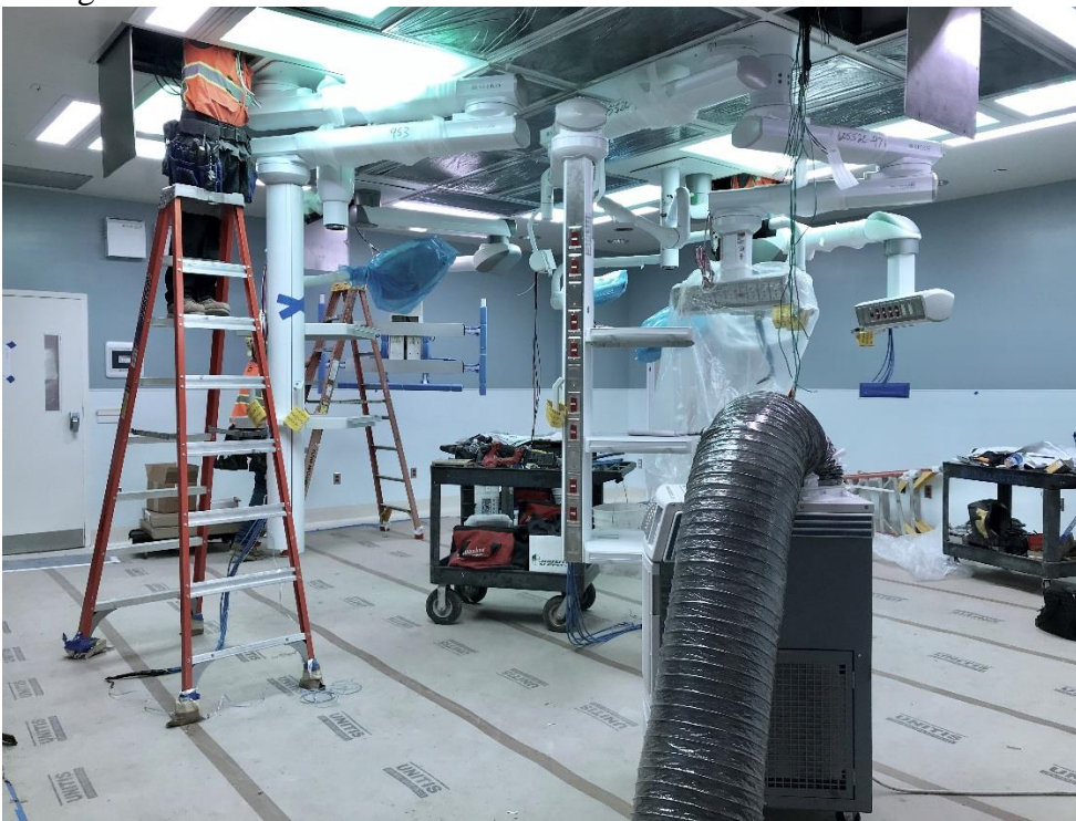
2-20-18: OR #1027 (Open Heart OR) Overhead Medical Equipment installed; working to install electrical, low voltage wiring.
