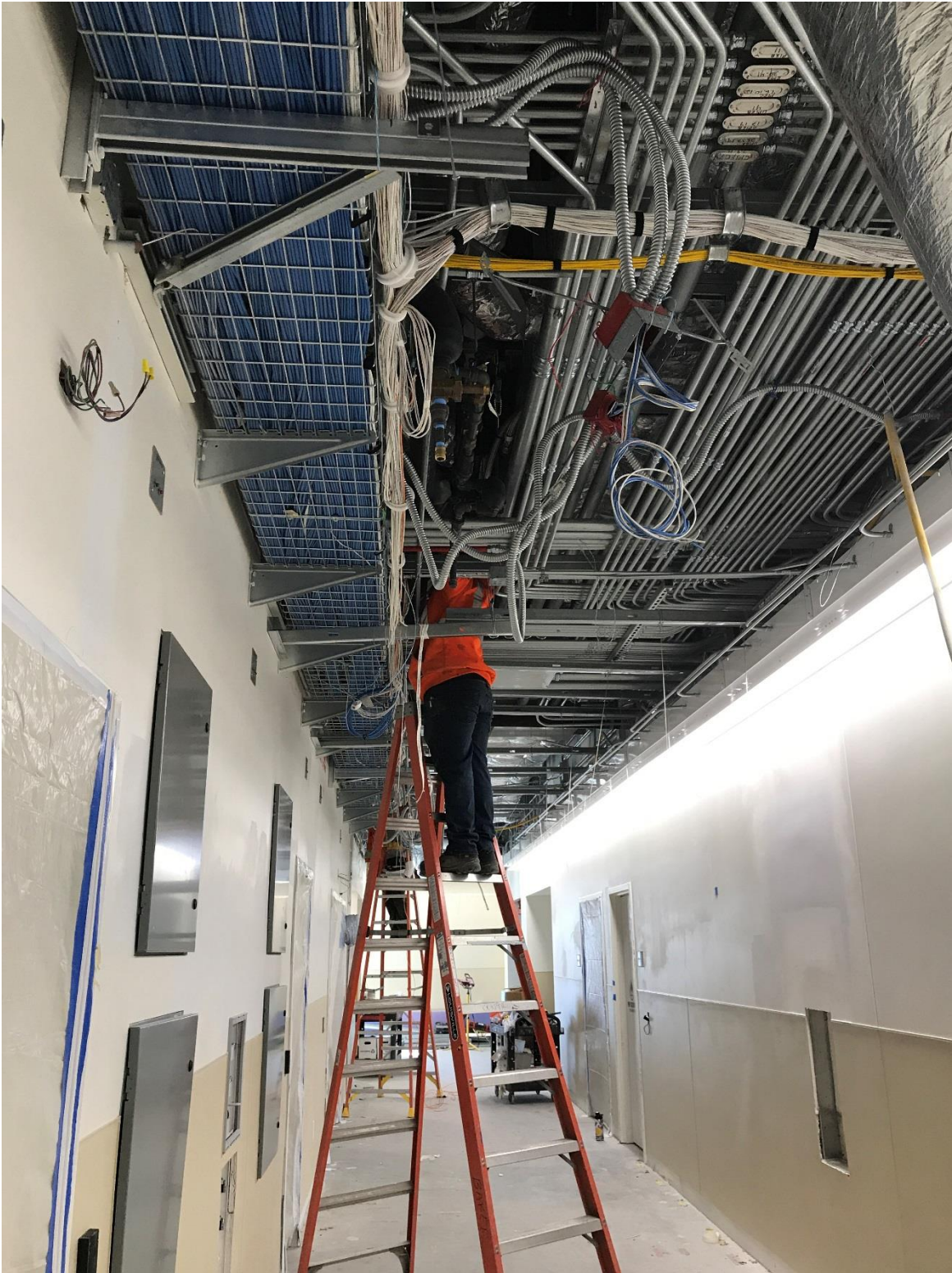
2-20-18: West Corridor: The finished ceiling will be installed at 9'-6" above the floor. Infrastructure in the form of plumbing piping, mechanical ductwork, electrical conduits and low voltage cable trays fills the space from the ceiling to the underside of the roof, at 17'-6" above the floor.
