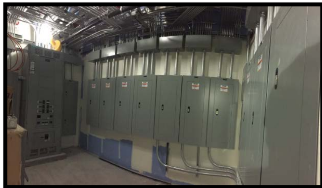
Level A Electrical Room
