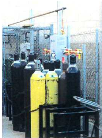
Tank Farm manifolds and new tank rack
